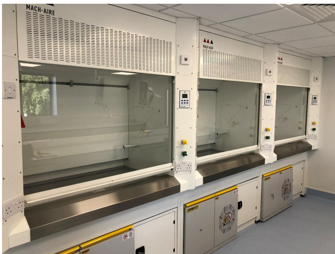
FUME CUPBOARD WITH FIRE RATED CABINETS BELOW
